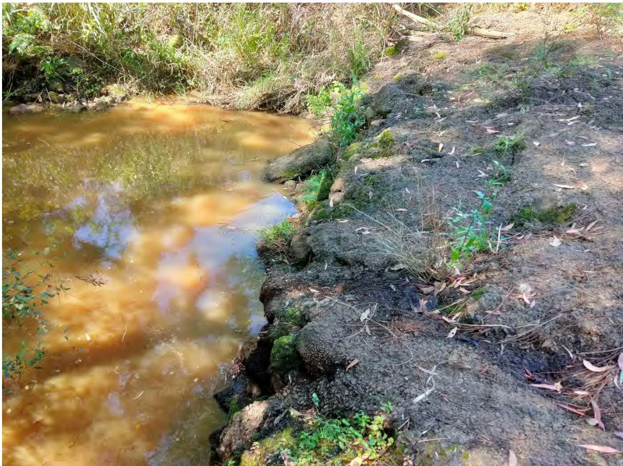
Plate 6 – The concrete apron on the downstream side of the pipes establishes a significant “drop structure”
