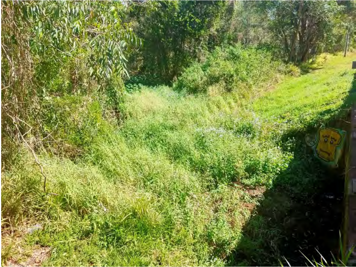
Plate 3 – Water ponds on the upstream side of the road, restricting fauna movement through the pipes
