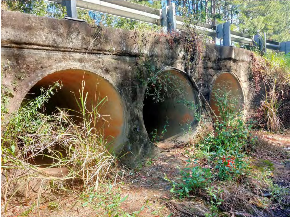
Plate 5 - 3 X 1500mm pipes convey the eastern tributary of Moogurupum Creek under Double Jump Road
