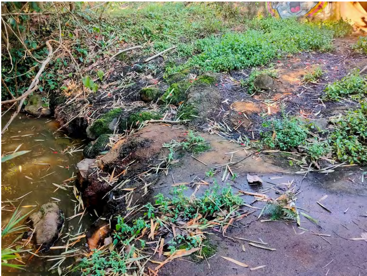
Plate 2 – The concrete apron on the downstream side of the pipes establishes a significant “drop structure”
